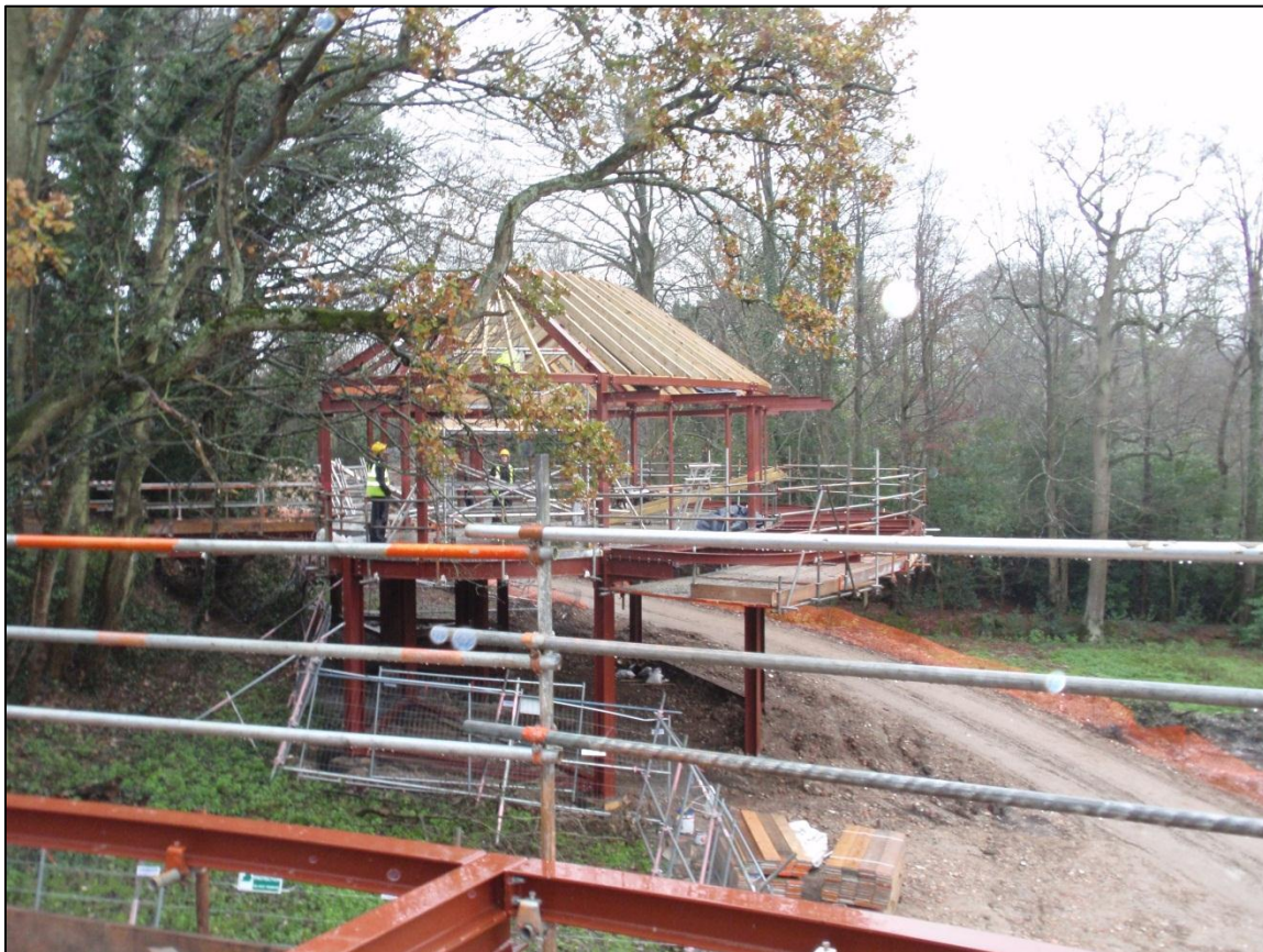
Assessing tree quality and demonstrating how the retained trees can be protected through construction activity is a busy area of work for UK expert witnesses.
