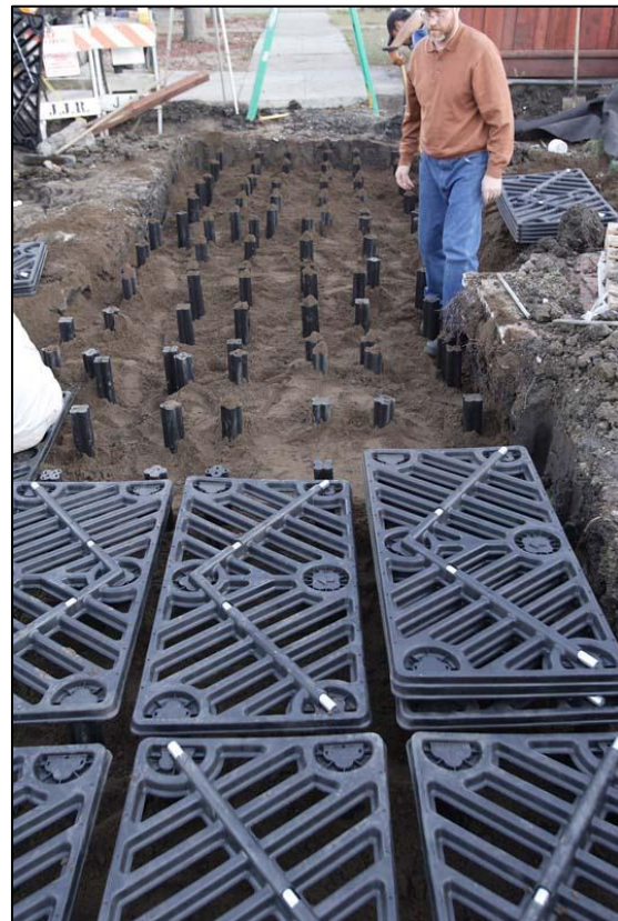
This Silva Cell installation in the US supports the finished concrete sidewalk on the reinforced cells, which allows tree roots to thrive in good quality soil beneath. The soil also acts as a temporary storage site when there are surges in rainwater runoff.
